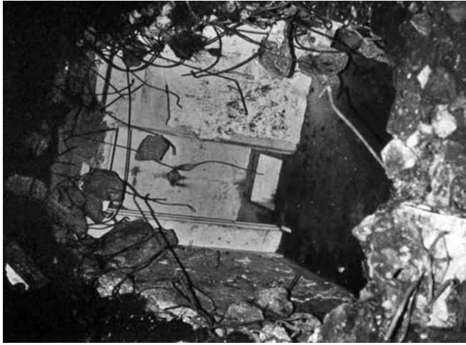
Part of the roof of the nuclear post broken into 'accidentally' by the contractors in 1979/80
